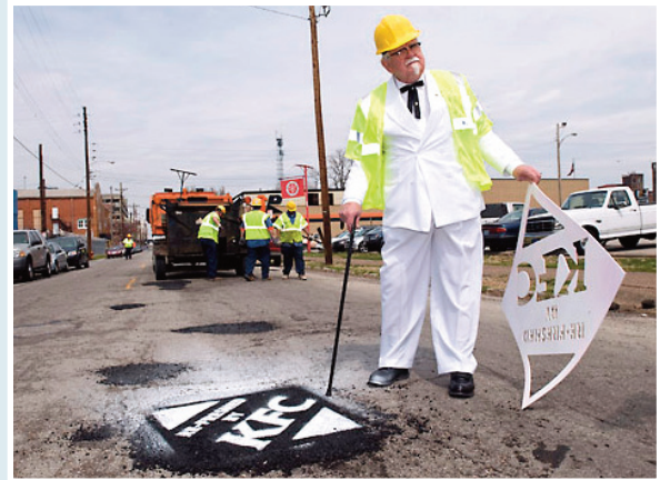
KFC recently paid for 350 potholes to be repaired in Louisville, KY
